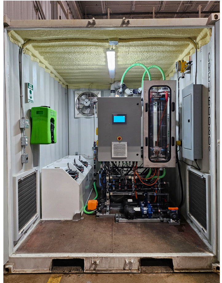
Axine's electraCLEAR™ pilot system on customer site
